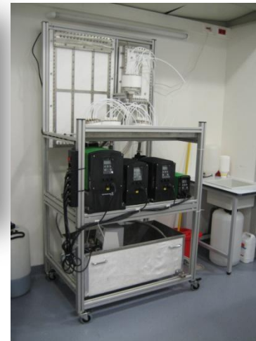
NETmix® pilot plant
